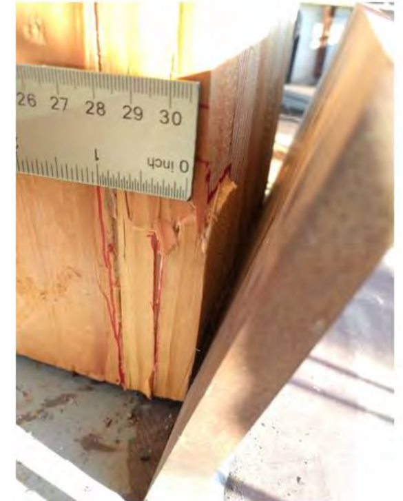
Chipping of wood at the rocking wall corner
