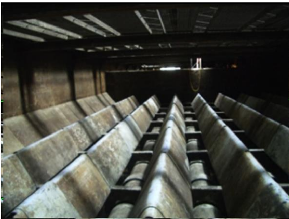
Baffle Boards, Moniwa WTP before the event.
