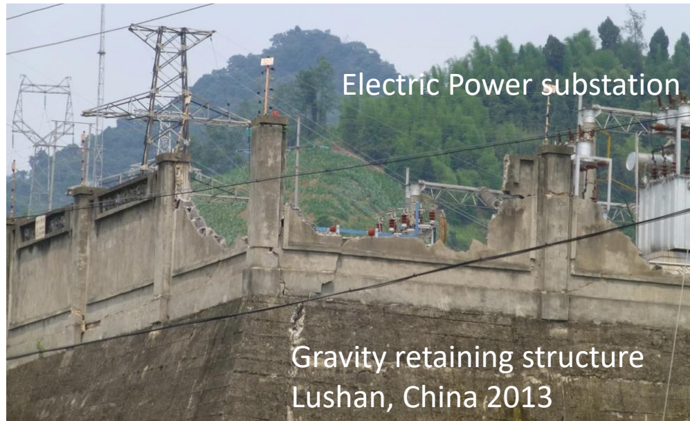
Gravity wall structure displaced
